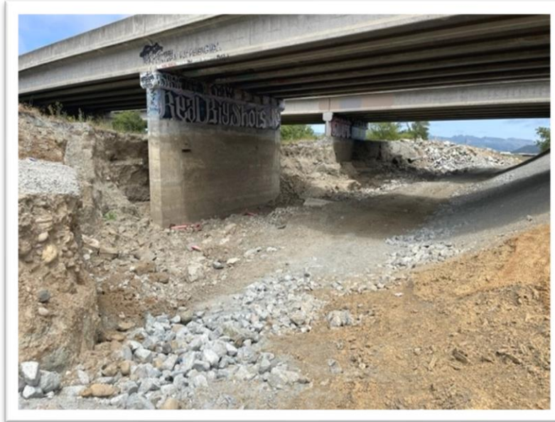
Figure 8. Erosion under Highway 1 from floodwaters overtopping and entering Willoughby Farms' Trafton and Cox Ranches.
