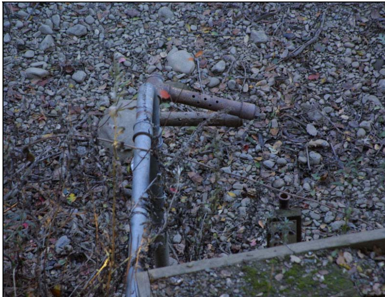
Figure 11: Intake and discharge pipes at Pacheco.
