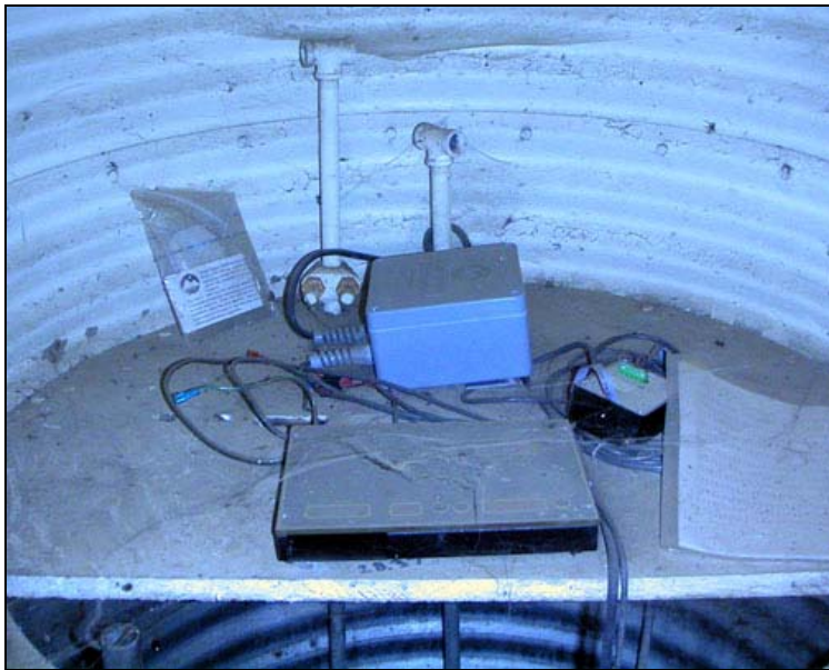
Figure 6: Pressure transducer equipment in a stilling well (Pacheco).
