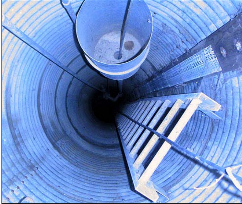
Figure 5: View inside of stilling well (Pacheco Creek).
